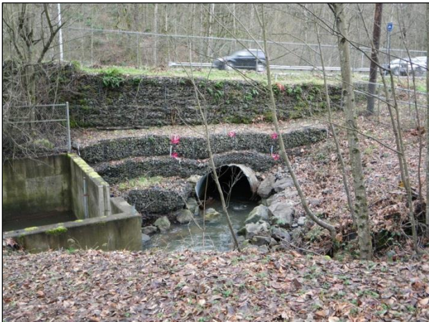
Deteriorated culvert upstream
