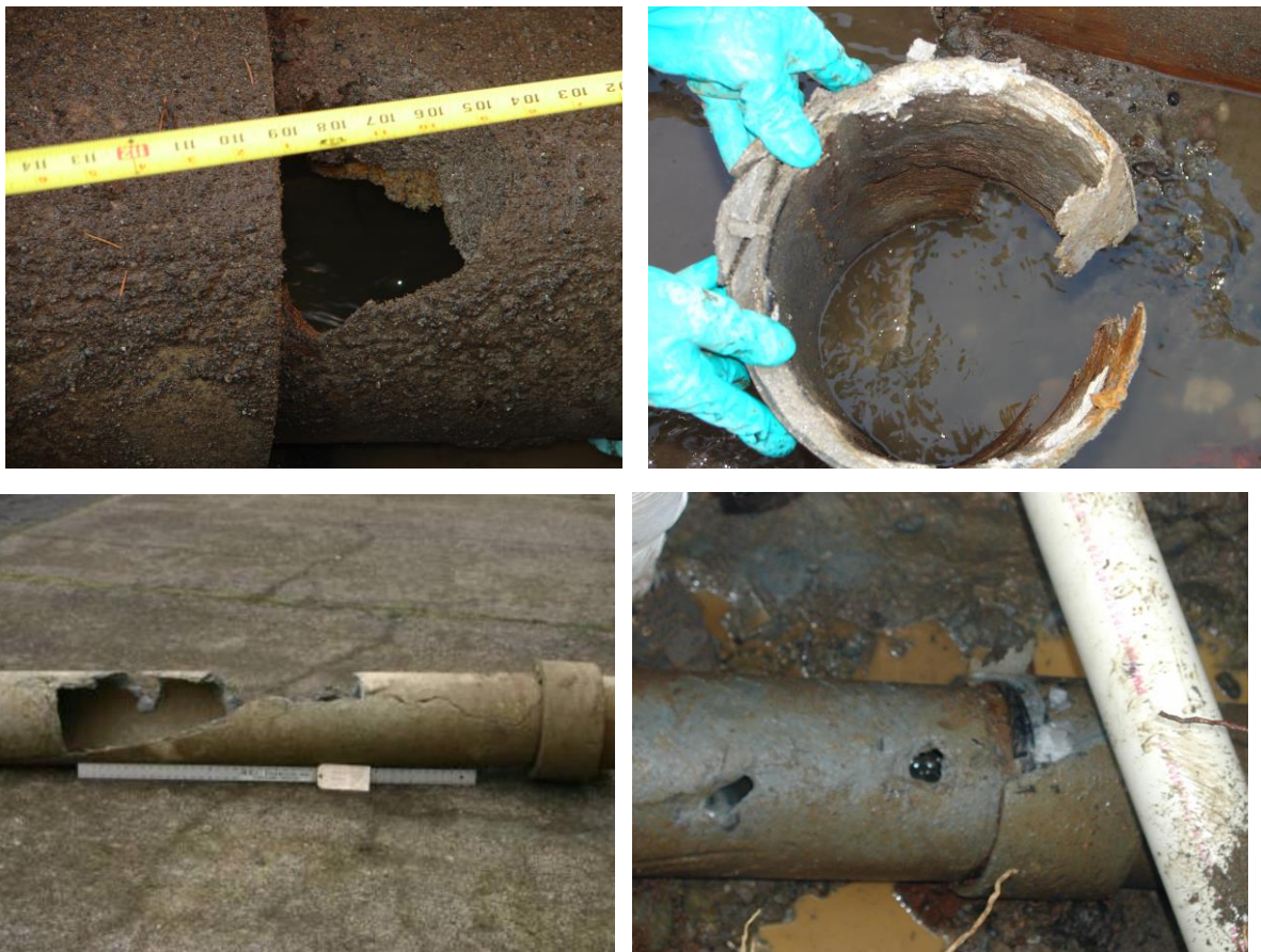
Figure 6-3: Meydenbauer Bay Lake Line Deterioration
