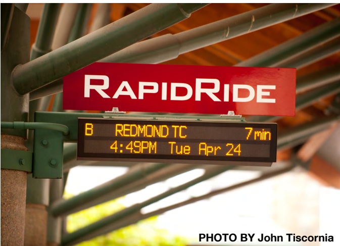
Figure 68 Real-time arrival information signboard installed by King County Metro at the Bellevue Transit Center for RapidRide B Line service.
