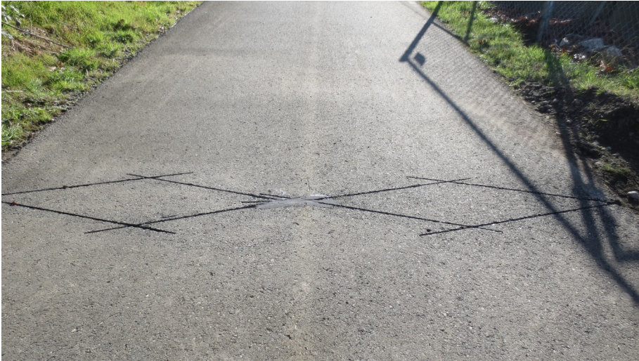
Inductive Loop Detector (SR-520 Trail)
