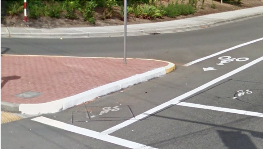
Bike lane inductive loop 145th Pl SE and SE 24th St intersection, southbound
