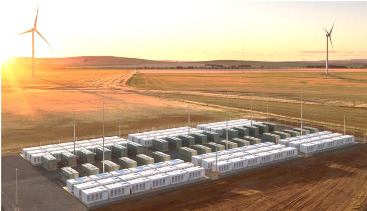
Figure 16: Hornsdale Power Reserve is 100MW/129MWh, approximately 43 times smaller than the Complete Solution 42
