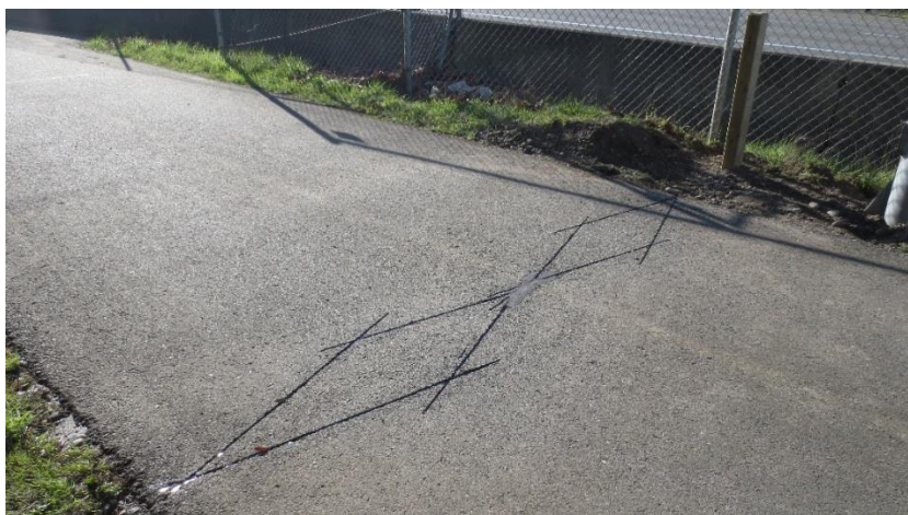
Inductive Loop Detector at SR-520 Trail
