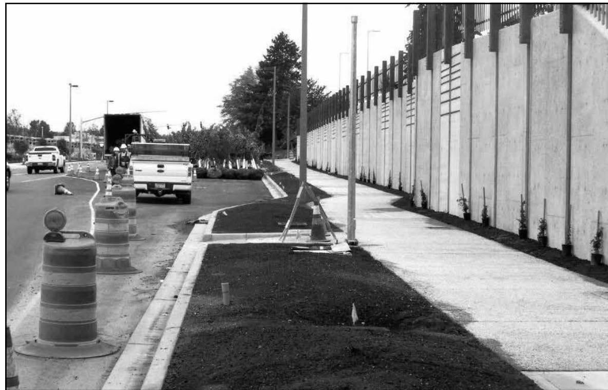
Improvements to 120th Avenue Northeast between Northeast Fourth and Seventh streets are nearly complete. The stretch between Northeast Seventh and 12th streets is now underway.
