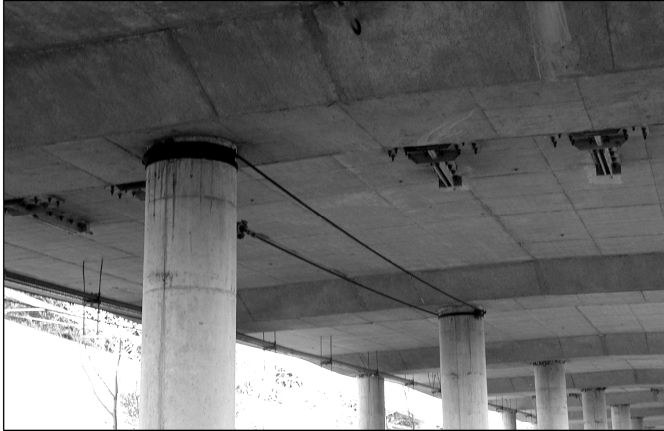
Figure 4. Cable restraint fabricated in 1987 across Joint #9 on 90/43WCD to prevent loss of bearing.
