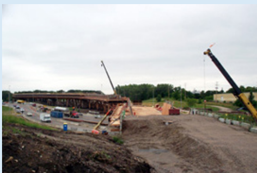
Construction of bridge crossing using hay bales and/or fabric filters runoff control strategies to minimize impact on surrounding land.
