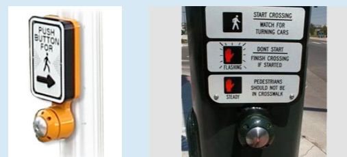
Accessible pedestrian signals incorporate large push-buttons that can be actuated by people with limited dexterity. Some models may include vibrotactile arrows and pedestrian instructions (Source: walkinginfo.org and www.mtc.ca.gov).
