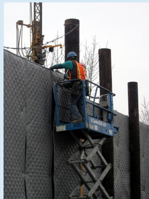
Installation of noise blankets at Beacon Hill Light Rail Station, Seattle. (photo courtesy Sound Transit)
