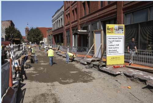
Business access signage for Mall Extension light rail construction, Portland, OR (Damian Conrad Photography)
