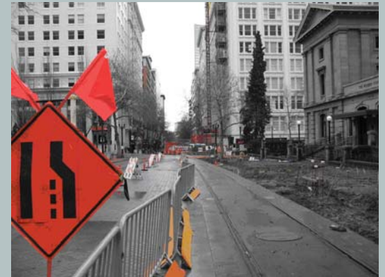
TriMet broke up the transit mall construction in Downtown Portland into short segments to reduce the duration of time construction took place in front of any one group of businesses.
