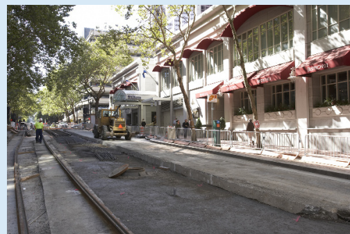
Access for pedestrians and businesses during light rail construction on the Transit Mall in Portland, OR (Damian Conrad Photography)
