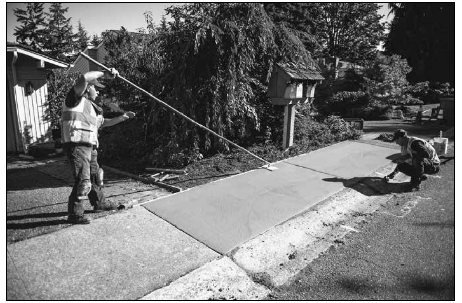
Neighborhood sidewalk projects like this one will be funded by the levy.
