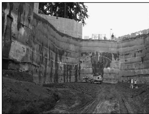
Tunnel excavation at the south portal (Main Street/112th Avenue Southeast) began in late January and will be going 24/7 as the sequential excavation method of tunneling requires a constant operation.
