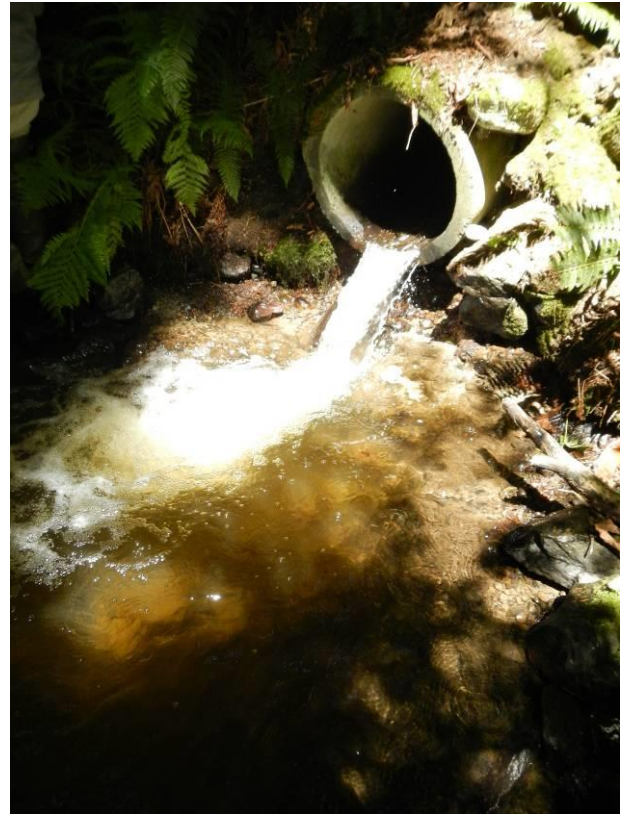
Top end of reach on Yarrow Creek RM 1.8 (notice culvert acting as hydrologic block)
