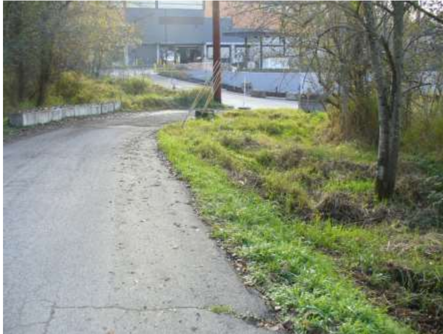
Photo 2 – Access road stream crossing location is near the concrete blocks on the left. 11/20/18
