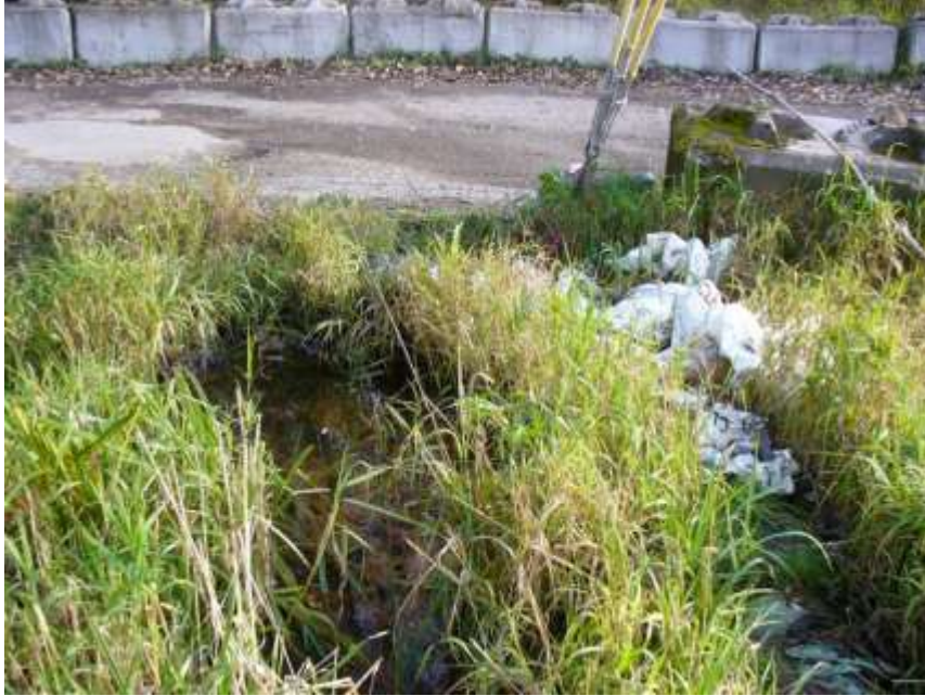
Photo 6 – Remnants of the sand bag streambank placed in the fall of 2016 are on the right side. This 11/20/18 photo shows that the water level at culvert outlet is high. Orangish iron bacteria indicating groundwater flow source can be seen (faintly) in the water, access road in the background.
