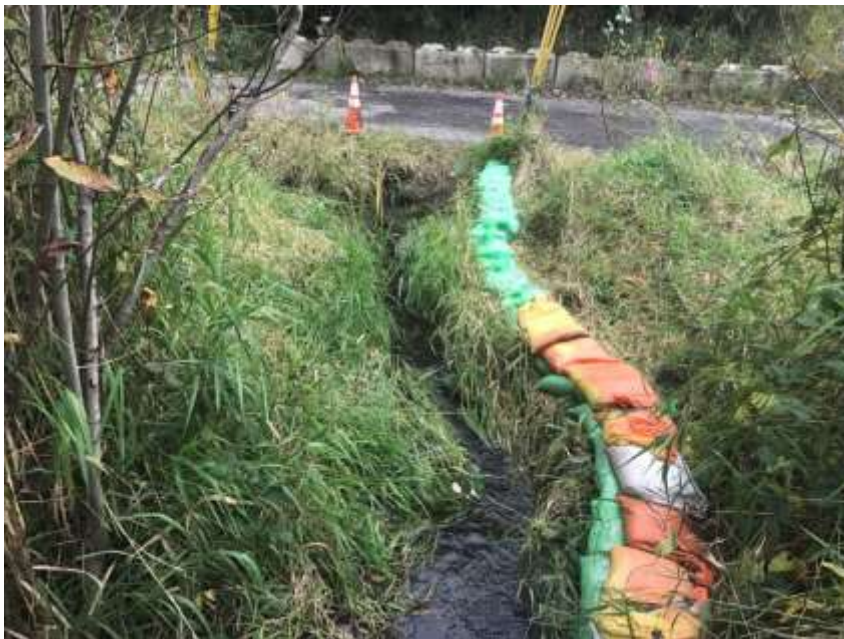
Photo 5 – Sandbagging has been used below the culvert outlet as a stopgap measure to keep (most) flows within the stream channel at normal flows. 10/19/16
