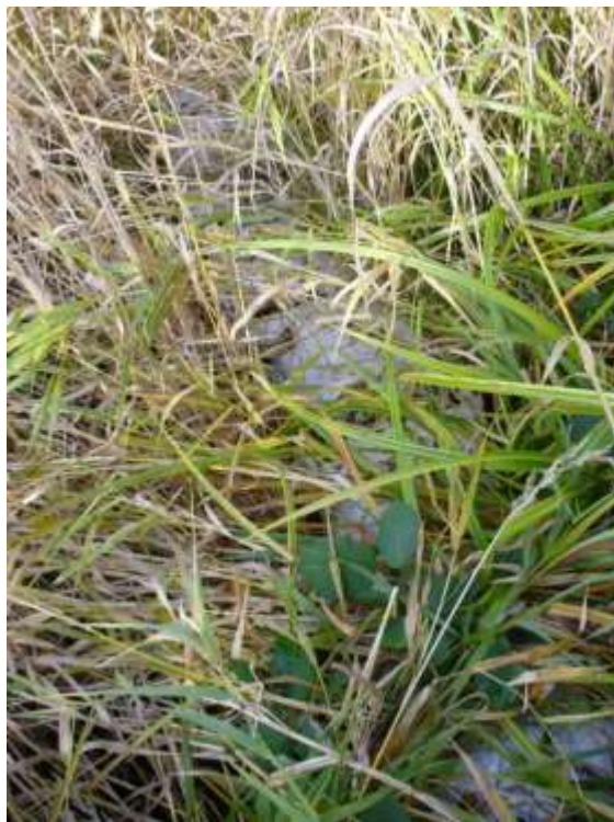
Photo 9 – Sandbags placed two years ago in 2016 are overgrown and deteriorating such that the sand is spilling out and the top of the barrier is lower, offering diminished protection. 11/20/18
