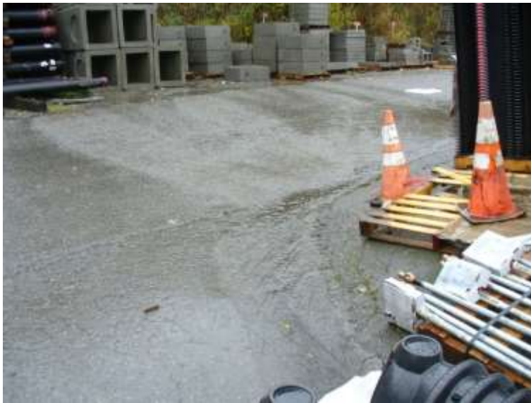
Photo 17 – Water from the hole in the wall in the previous photo sheet-flowing across the Fowler yard. 11/26/18
