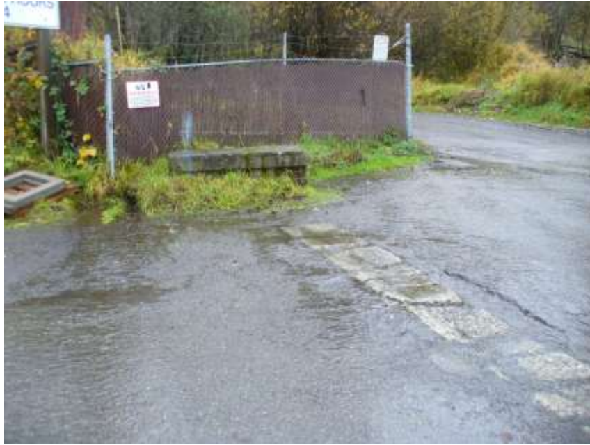
Photo 14 – Water spilling out of the channel just downstream of the access road flows across an access drive to the Fowler yard off of SE 30 th , shown here, then continues westward along the north side of the road. 11/26/18
