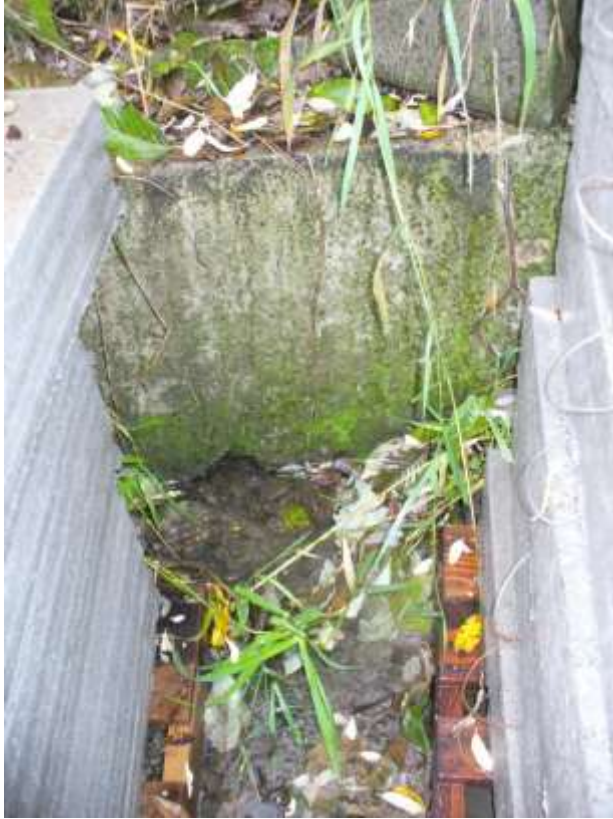
Photo 16 – Pictured is a hole in the ecology block wall separating the stream channel from the Fowler yard – with water flowing through. 11/26/18
