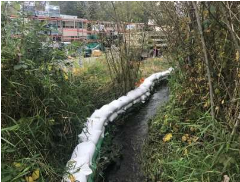
Photo 7 – Sandbagging extending farther downstream from the culvert outlet in an effort to keep flows from spilling into the Fowler storage yard. 10/19/16
