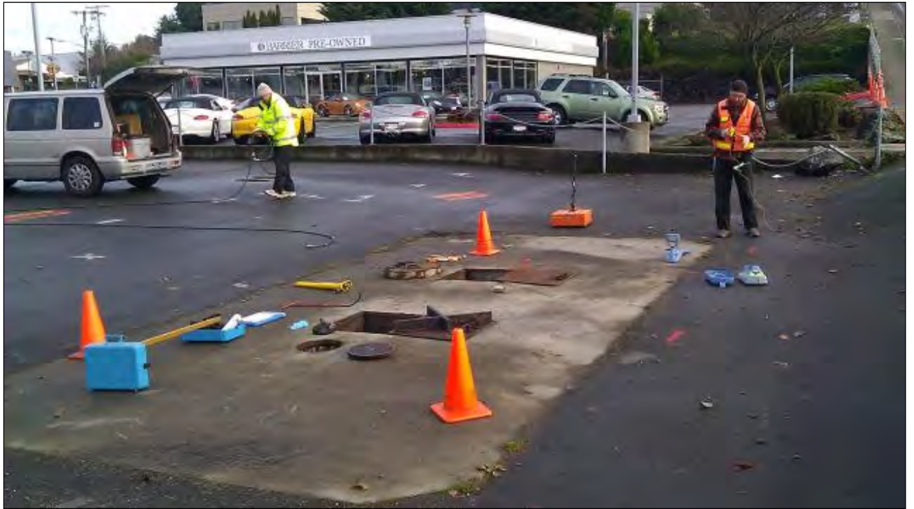
Geophysical survey crew working on Triangle Parking Lot. UST beneath concrete pad in foreground – Looking East
