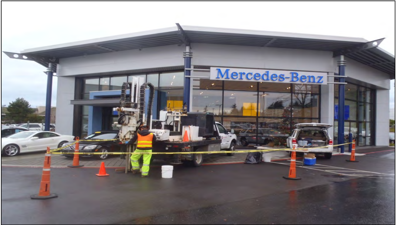
Drilling at the Barrier Mercedes Lot property to complete B-119E boring – Looking East
