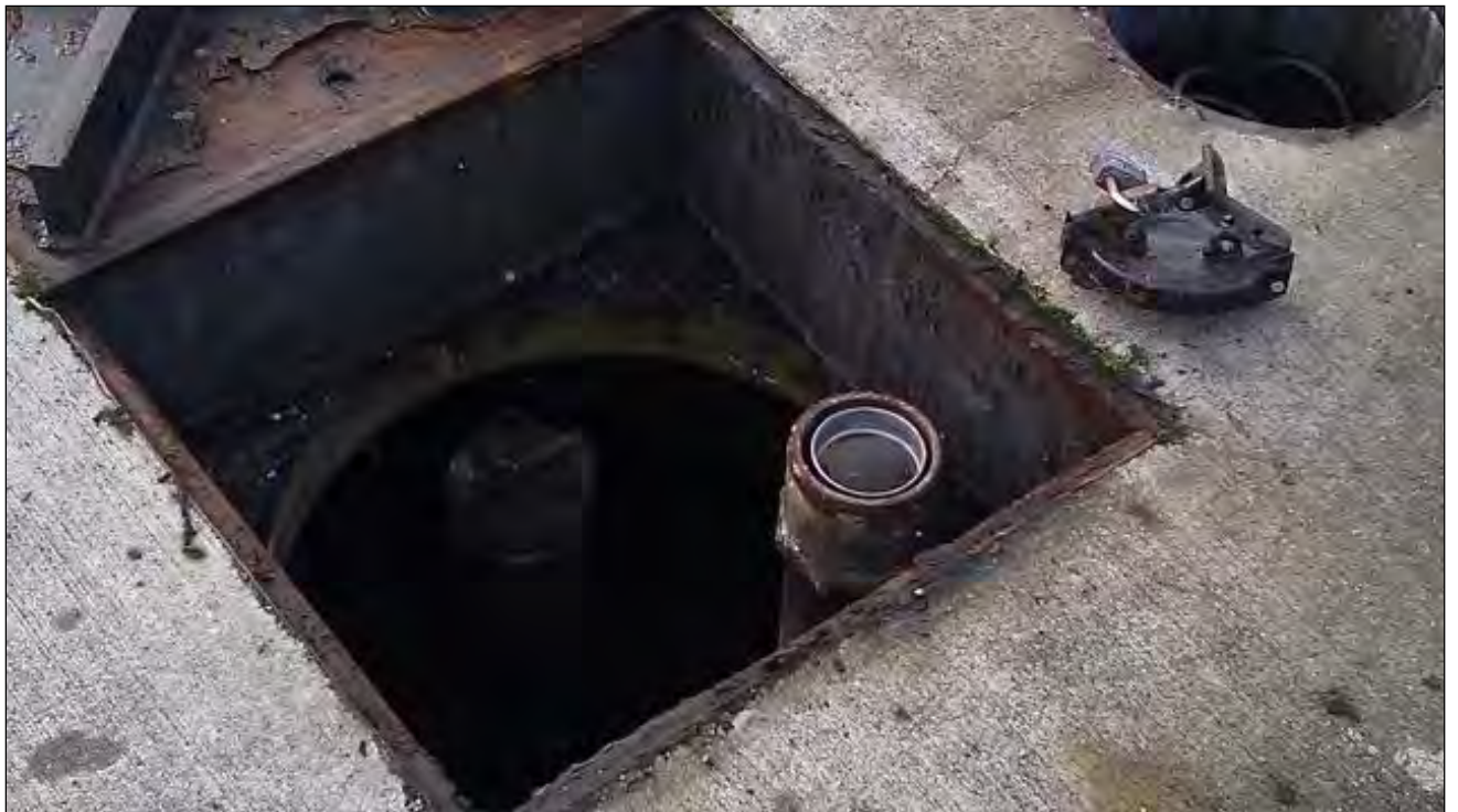
Apparent UST fill port observed within the vault
