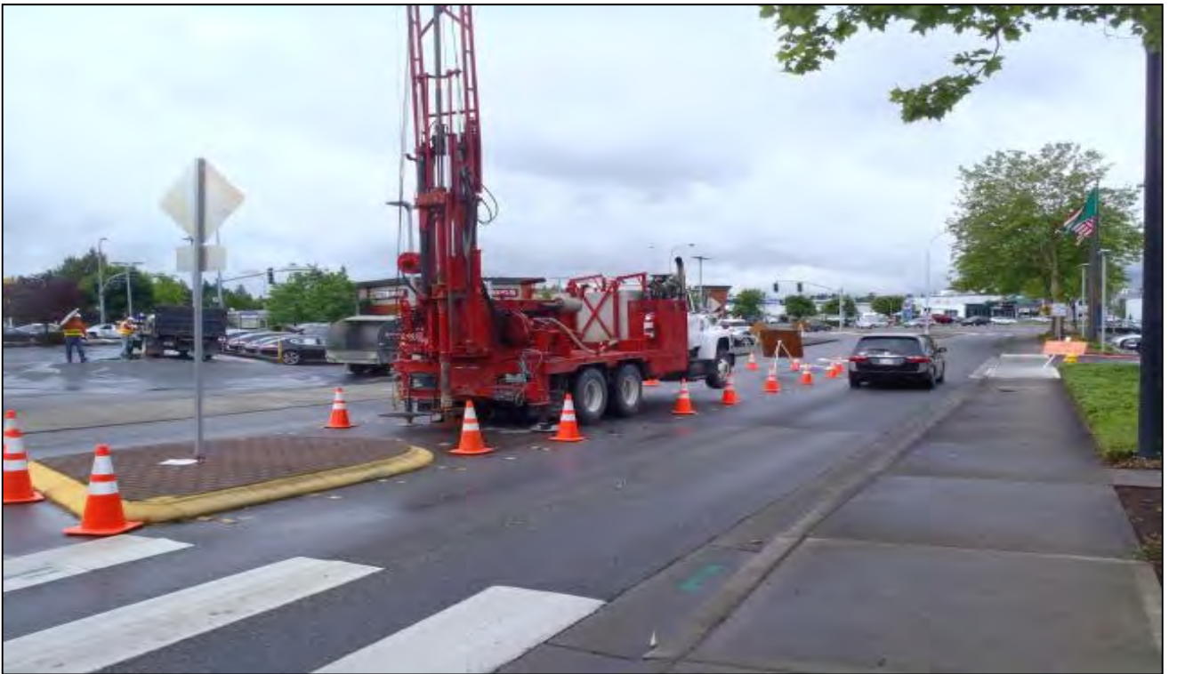
Drilling to install monitoring well GEIWMW-1 in center lane of Bel-Red Road - View to SW
