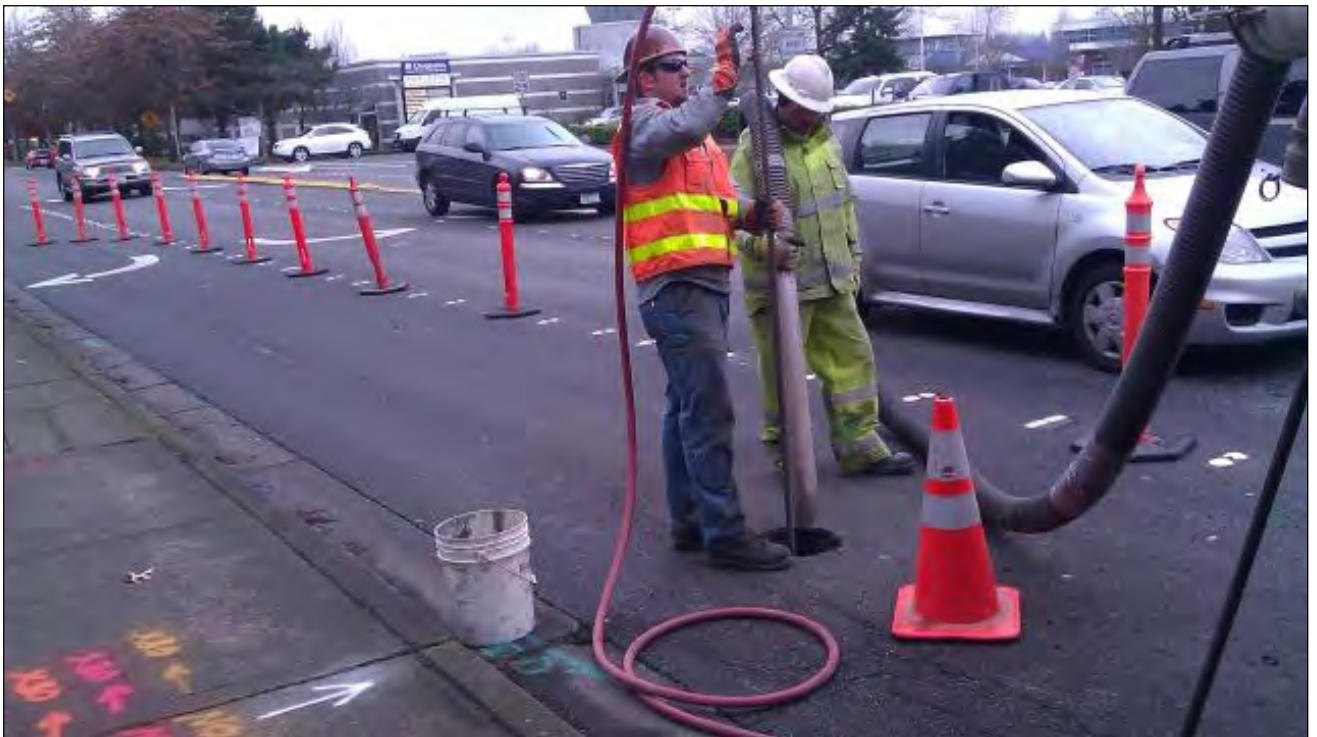
Traffic control and air-knife activities at boring B-101E in 120 th Avenue NE – Looking Southwest
