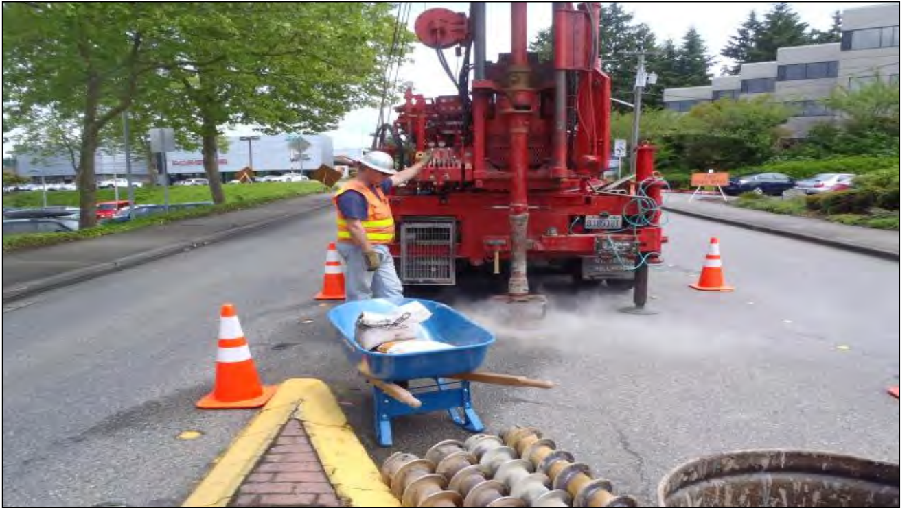
Drilling to install monitoring well GEIMW-2 in center lane of Bel-Red Road – View to East
