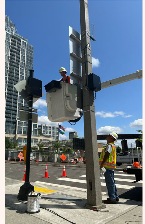
Figure 10: The first C-V2X system at an RRFB, in front of City Hall.
