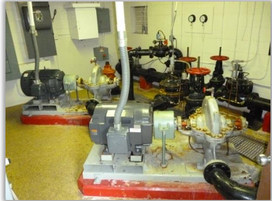
Existing Horizon View #1 Pump Station
