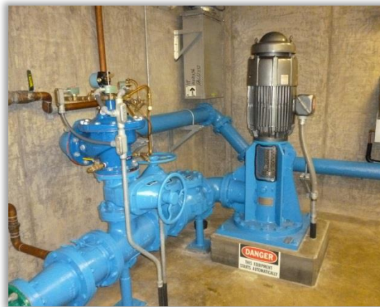
Meydenbauer Pump Station
