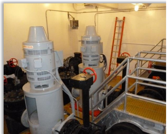
NE 8th Inlet Pump Station
