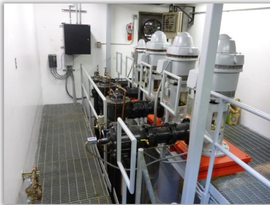
Existing Clyde Hill Pump Station
