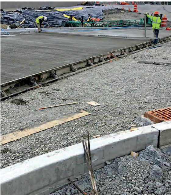
124th Avenue NE improvements between Bel-Red Road and Northup Way continue on schedule.
