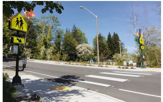
Example of a Rectangular Rapid Flashing Beacon installed at a crosswalk.
