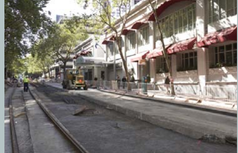
Access for pedestrians and businesses during light rail construction on the Transit Mall in Portland, OR. (Source: Damian Conrad Photography)
