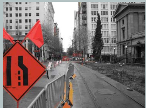
Staggered construction in downtown Portland reduced duration of construction in front of any one group of businesses. (Source: City of Bellevue)
