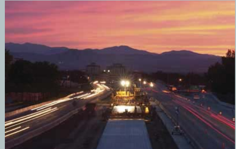
To reduce traffic and noise impacts to businesses, a significant amount of demolition and major reconstruction work for the T-REX project occurred at night. (Source: T-REX Project).
