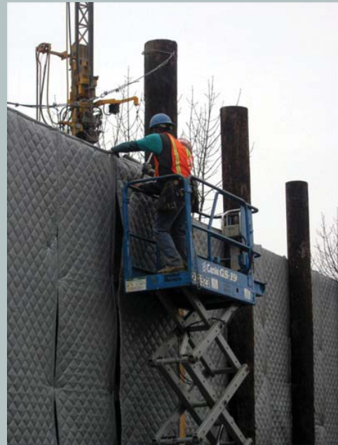
On Beacon Hill, Sound Transit installed noise absorbing materials on walls surrounding a construction staging area to reduce impacts on the surrounding community. (Source: Sound Transit)
