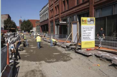
Business access signage for Mall Extension light rail construction, Portland, OR. (Source: Damian Conrad Photography)
