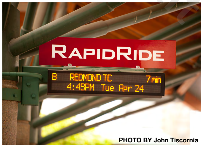
Figure 65 Real-time arrival information signboard installed by King County Metro at the Bellevue Transit Center for RapidRide B Line service.
